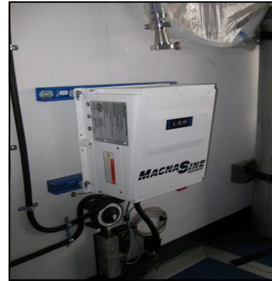
inverter/charger converts AC to DC battery power
