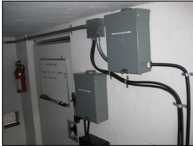
breaker panels for AC input and internal power distribution
