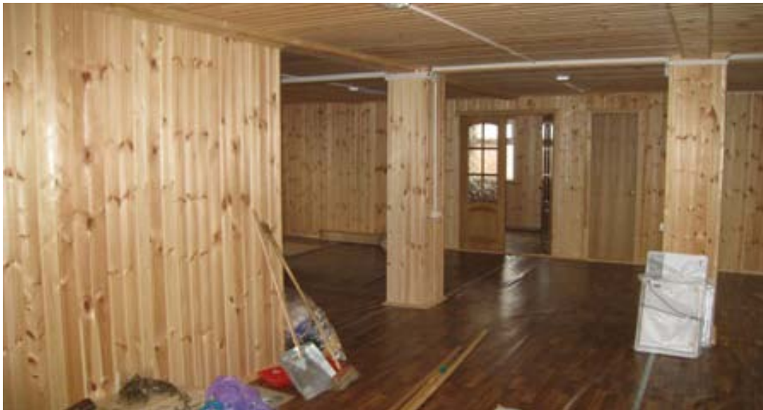
Figure 4.4 Interior of the Clean Air Facility in September 2009
