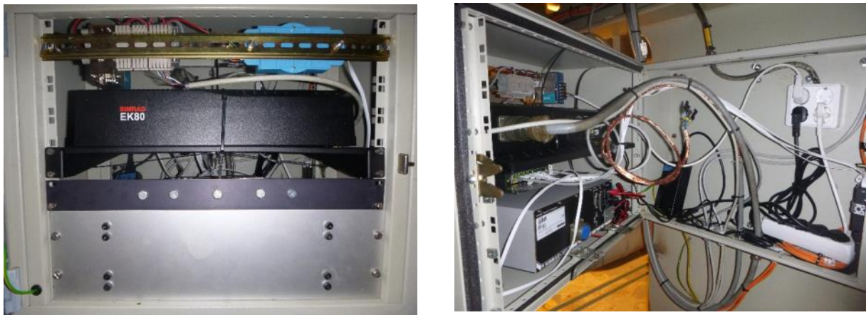
Figure WC-3: EK80 WBT installed in rack with EK60 GPT in tween deck below gym. Left – front view of rack with front door open – GPT is behind gray panel on bottom. Right – back view with back door open – GPT on lower level – WBT on upper level.
