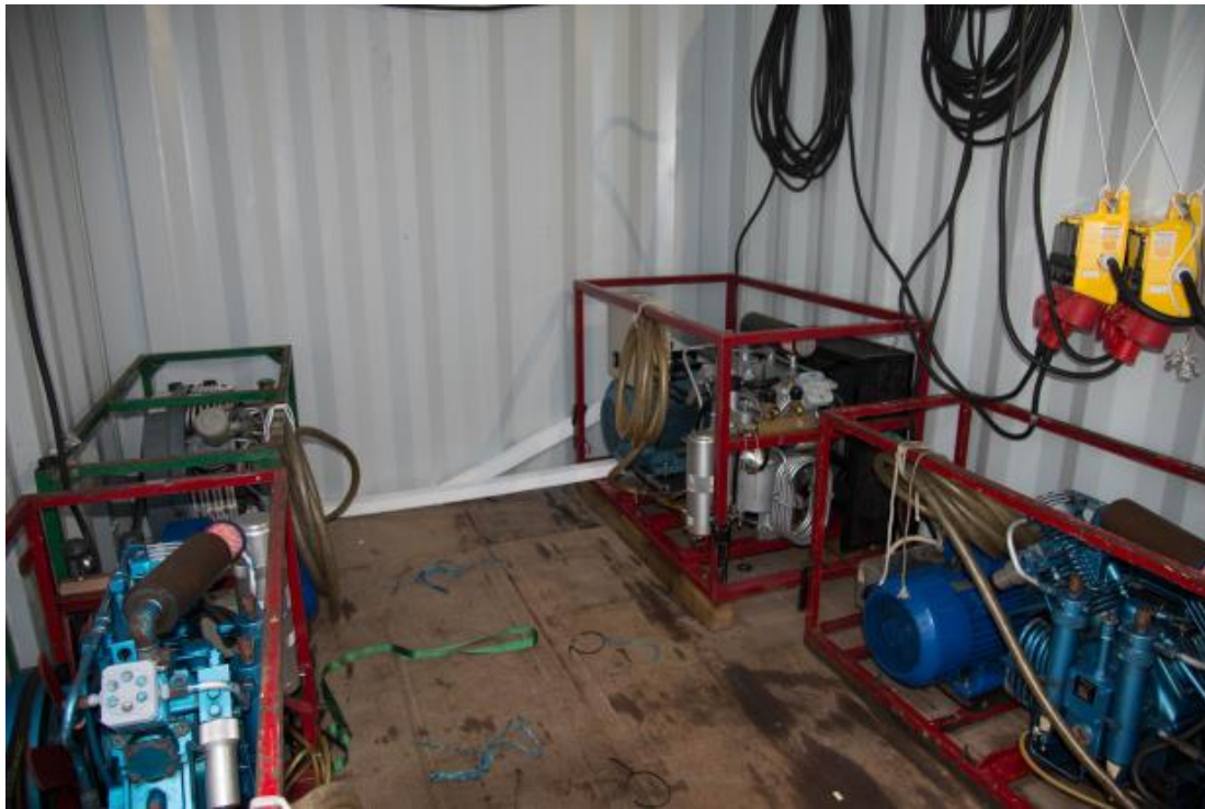
Figure GM-8: Air compressor used for air-supply to the seismic airgun.
