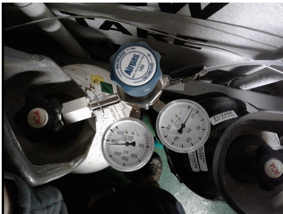
Pic 12: O2 regulator with shut off valve
