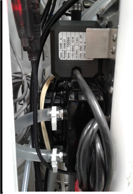
Pic 14: Water pump and fan+radiator.
