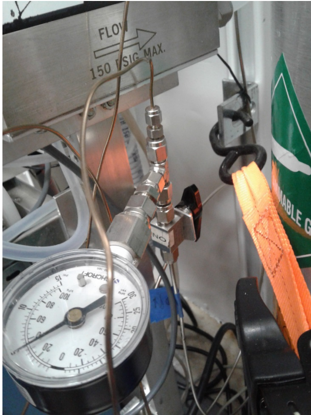
Pic 12: NO Shut off valve + NO pressure gauge
