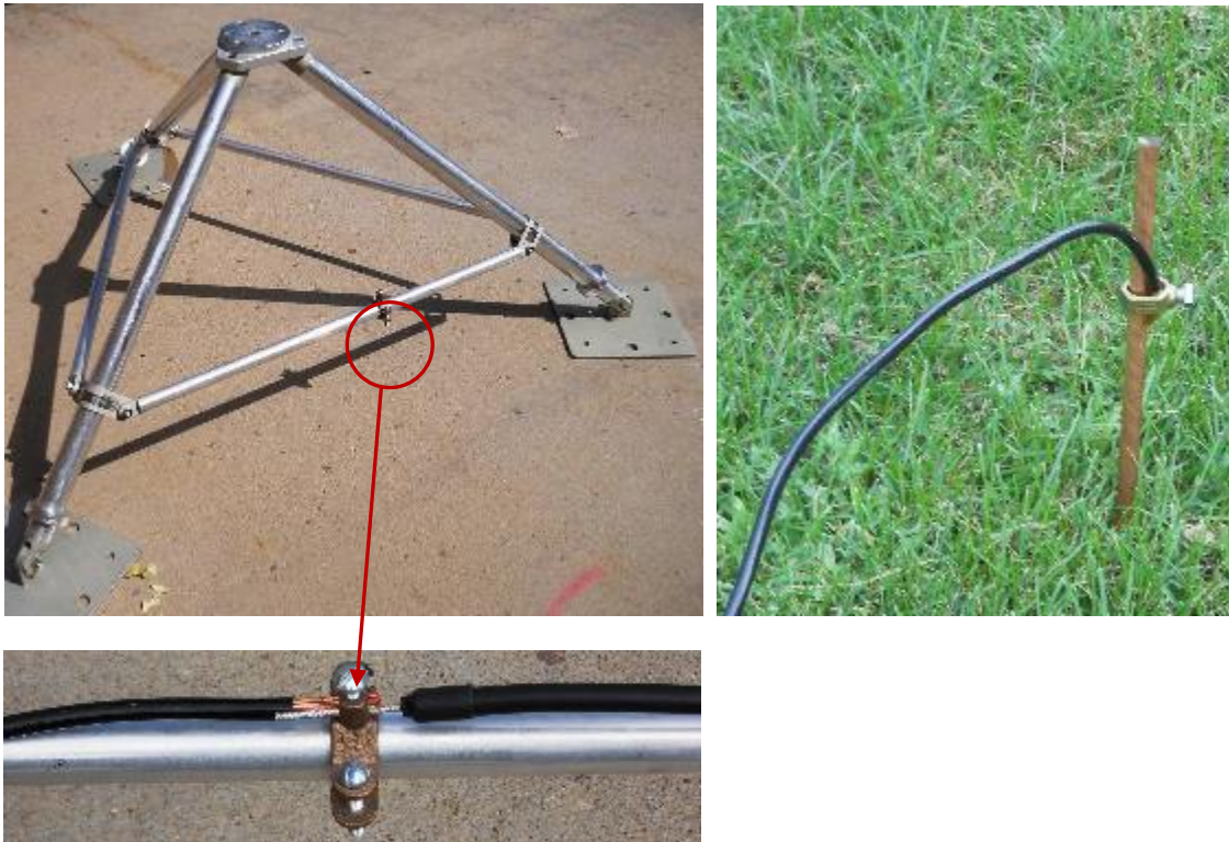
Figure 3-4. Tripod with clamp (upper left), close up of clamp (lower left), cable-to-Earth ground (right)
