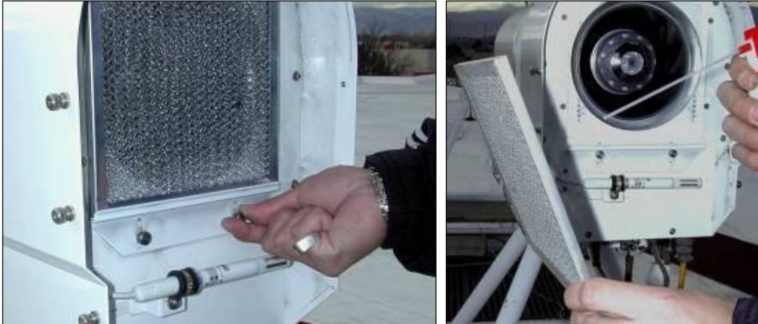
Figure 6-15. Superblower filter removal and cleaning
