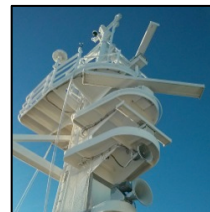
Rutter radar antenna (center)
