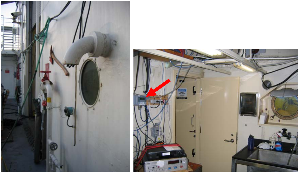
Figure A 3. Left: Inlet tube of the KM pressure sensor. Right: Location of the pressure sensor in the aft laboratory (lab#1).
