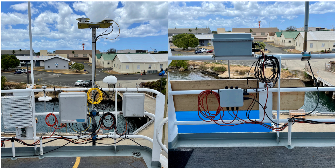
Figures 2-3: Pilot house roof installations: Radiometer mount, mean met and network switch boxes; heading box and power distribution box.
