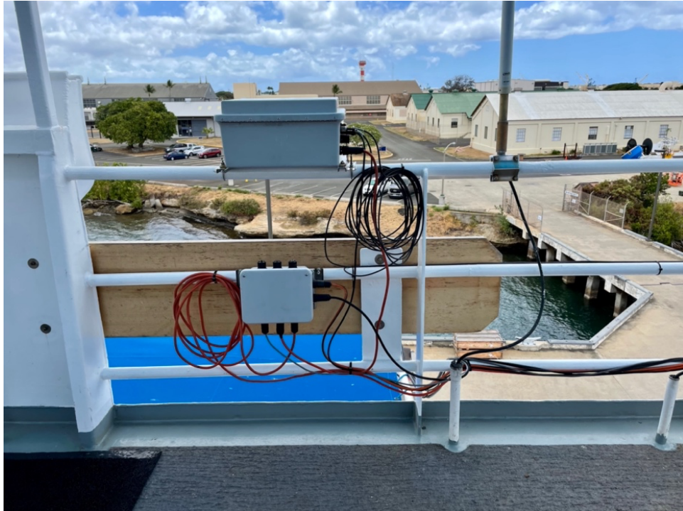
Figure 2: Heading system box and power distribution box, mounted on starboard side railing on the pilot house roof.
